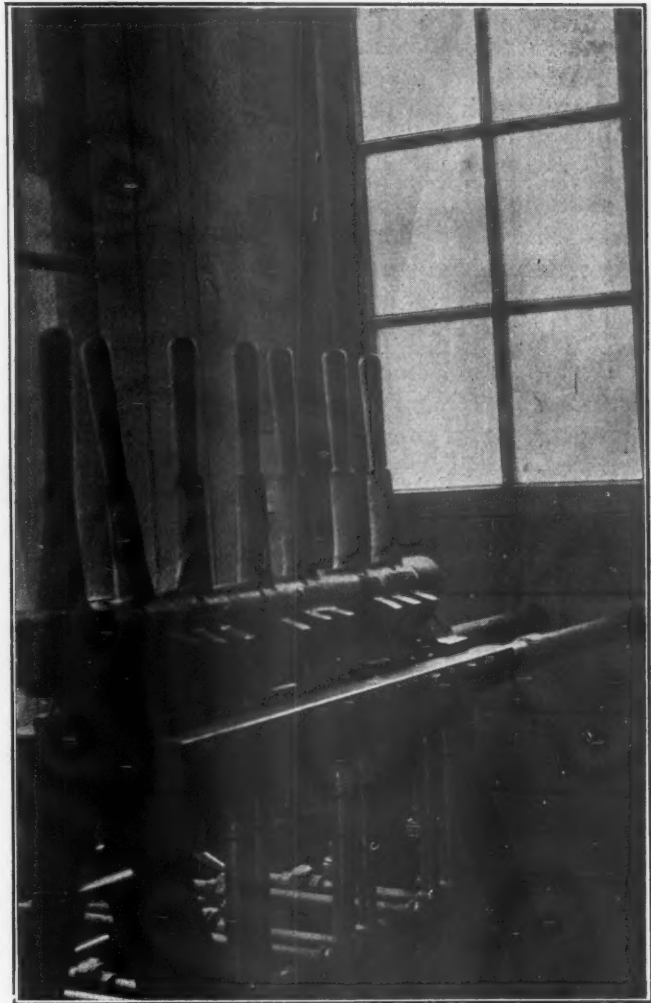
Air Control Levers at Top of One of the New Steel Towers
